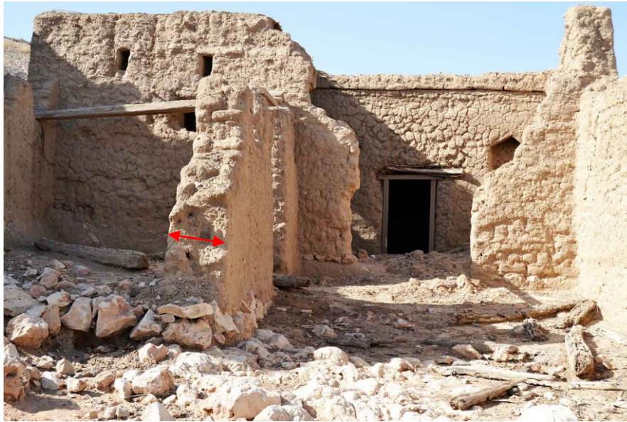
Picture 13: The width of external wall in traditional building was commonly varied from 40-80 cm
